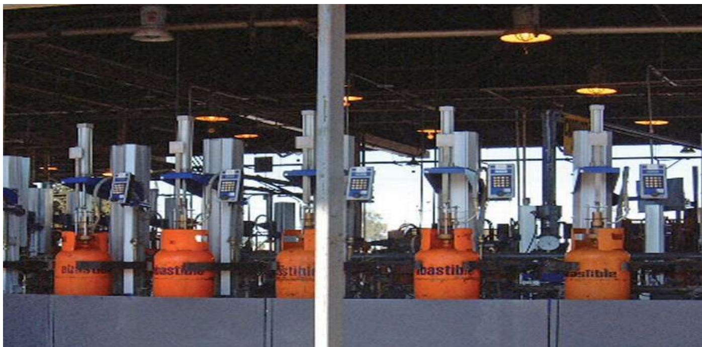
An automated carousel for filling of LP Gas Cylinders
