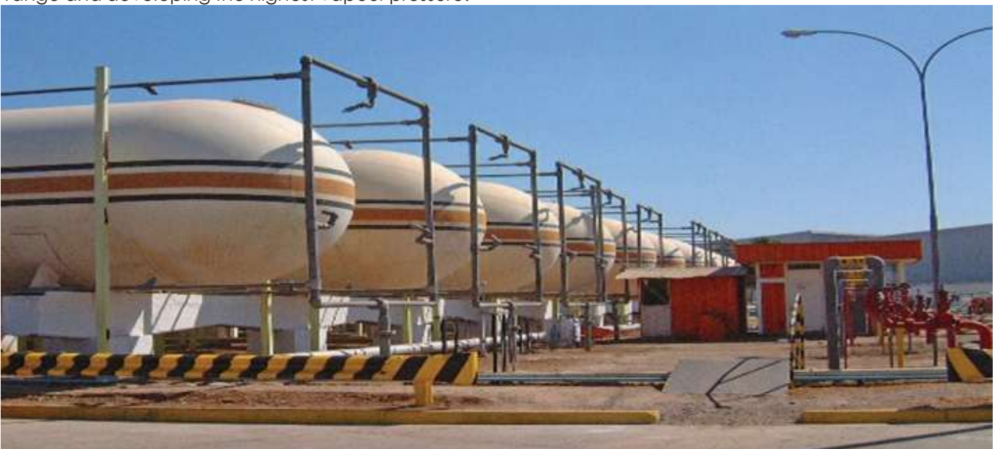
Above-ground cylindrical tanks for storage of LP Gas
